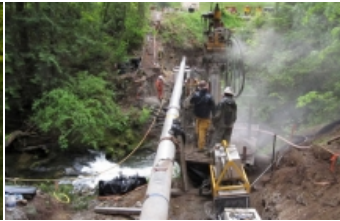
GeoEngineers designed micropile foundations (drilling shown here) that supported the structure and reduced its footprint.
