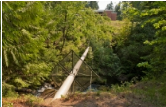
Potential threats to the exposed pipeline (shown here, before construction) included tree fall or gunfire.
